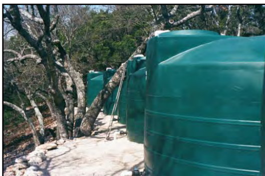
Figure 2-6. Low-profile 5,000-gallon polypropylene tanks
